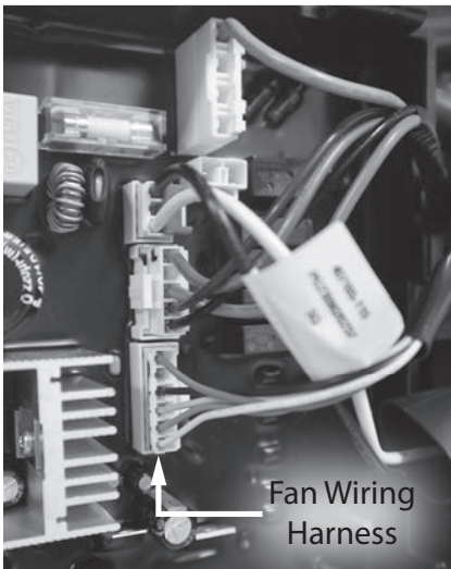
Figure 110 - Locate fan wiring harness on control board
