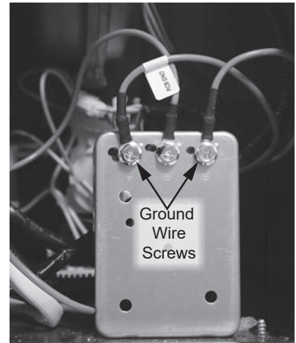
Figure 58 - Location of ground wires
