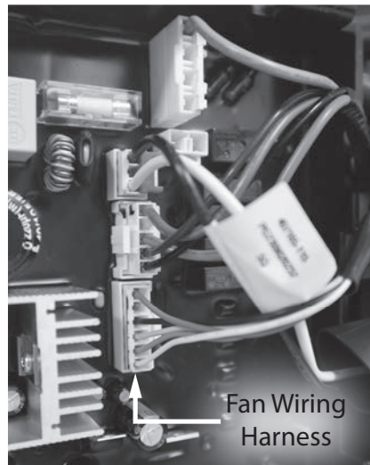
Figure 84 - Locate fan wiring harness on control board
