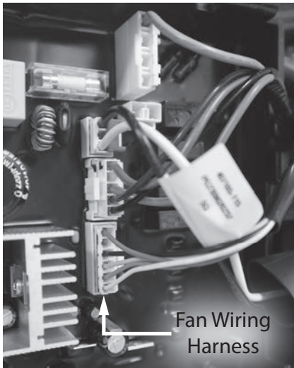
Figure 129 - Locate fan wiring harness on control board
